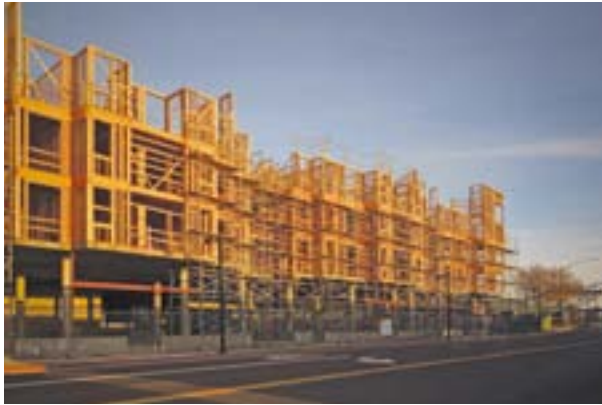
Construction in 2014 of a large four-storey apartment building near San Francisco, California, with three stories in timber construction atop a one-storey RC parking garage. © Randolph Langenbach
